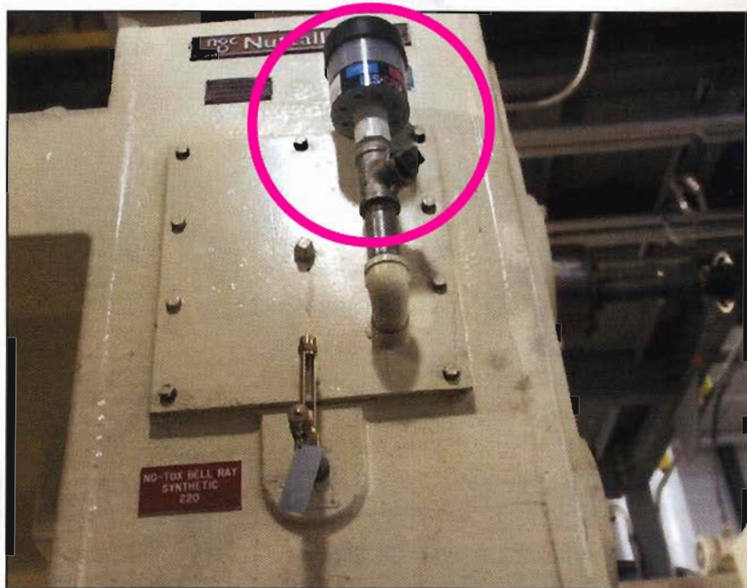
Figure 2. Sight glass added with oil sample port combo, desiccant with stainless piping and top-off plug between gearbox and desiccant.
